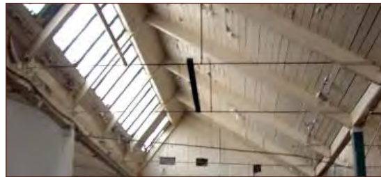
The interior of this manufacturing building illustrates the unusual saw-tooth roof system and windows providing a unique interior space.
