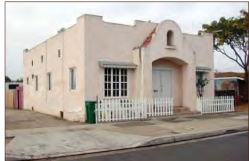
The rehabilitation of the former Friendly Center community center should include the restoration of the original bell tower and front doors.
