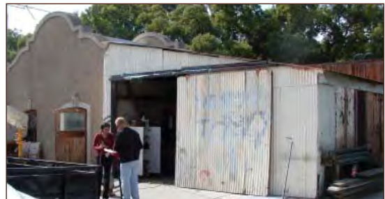
This inappropriate metal addition should be removed and any new addition should be compatible with the historic materials, size and scale of the original building.
