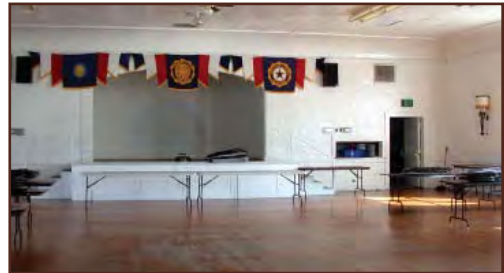
Significant interior features include the lodge hall stage, textured wall surfaces and wooden floor. Removal of the modern ceiling tiles and florescent fixtures would help restore the hall to its original appearance.
