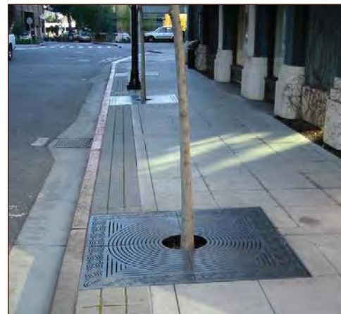
Active commercial and mixed use areas will have street trees in cutouts and/or tree grates.
