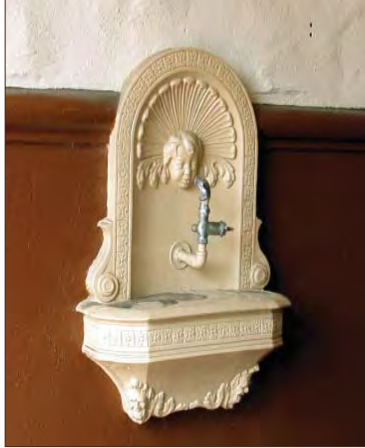
The decorative fountain in the lodge's recessed entrance is a distinctive feature that should be preserved and maintained.
