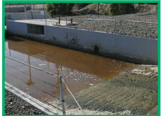
Example of a concrete water collection basin built wide enough to accommodate equipment to remove sediment.
