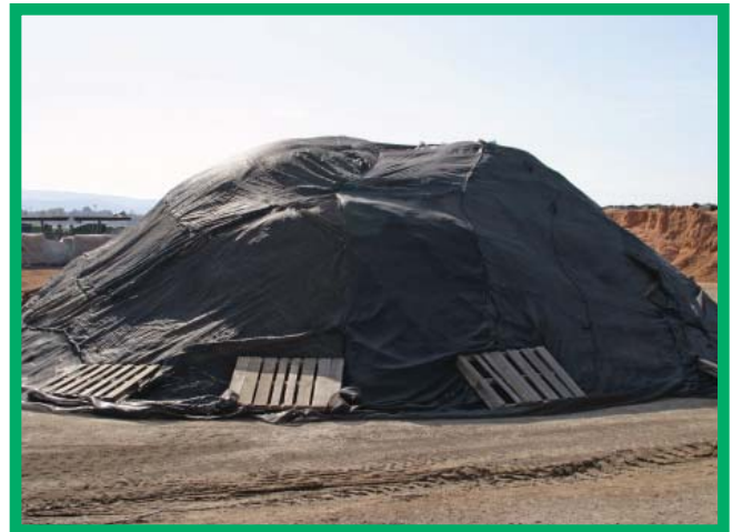
Example of soil pile covered with tarp to protect from wind and rain.
