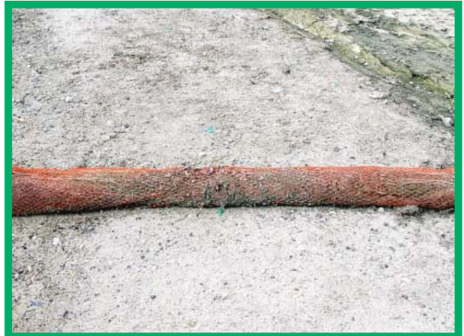
Example of a straw wattle placed around the perimeter of a compost pile to minimize movement of soil and associated pollutants during storm events.
