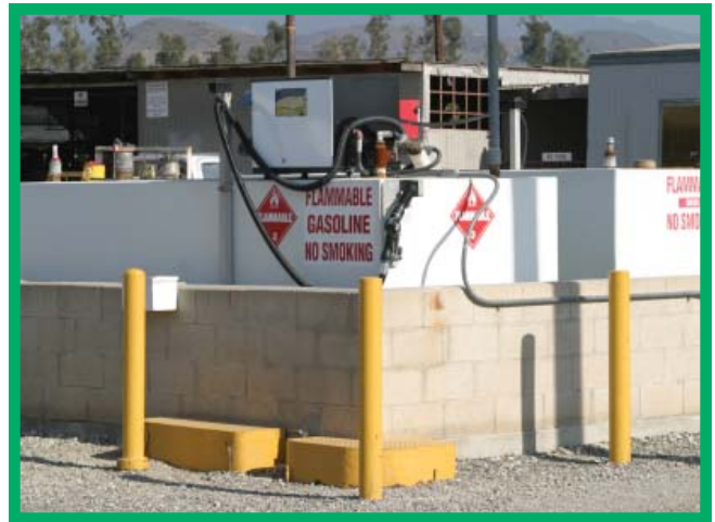
Example of a secondary containment area for containing fuel spills.
