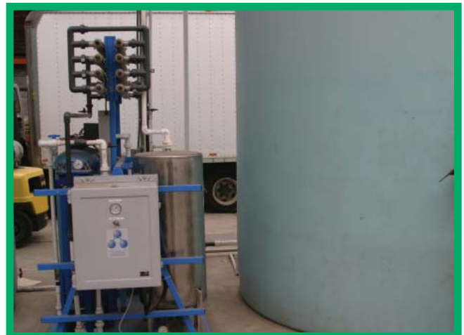
Example of an ozone treatment system.
