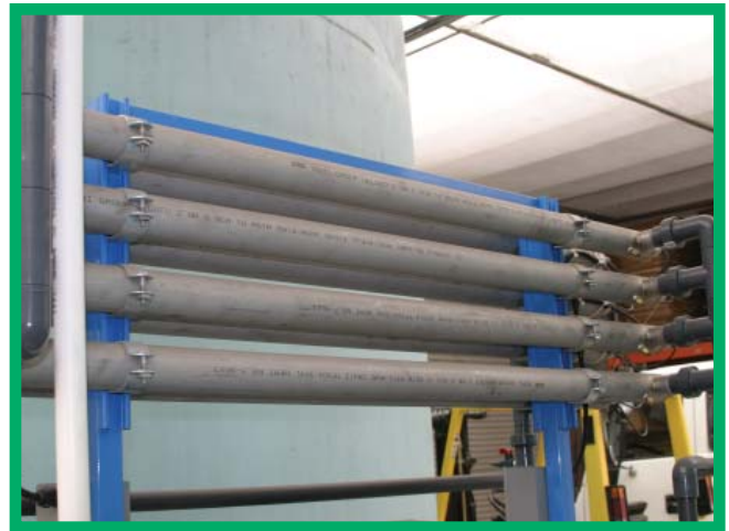
Example of an ultraviolet(UV) treatment system.
