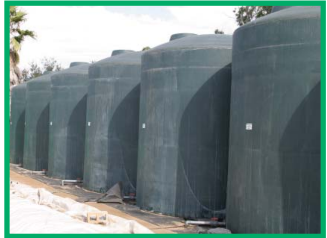
Example of a series of water storage tanks.
