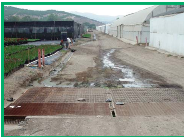
Example of sediment trap installed in road to trap sediment.
