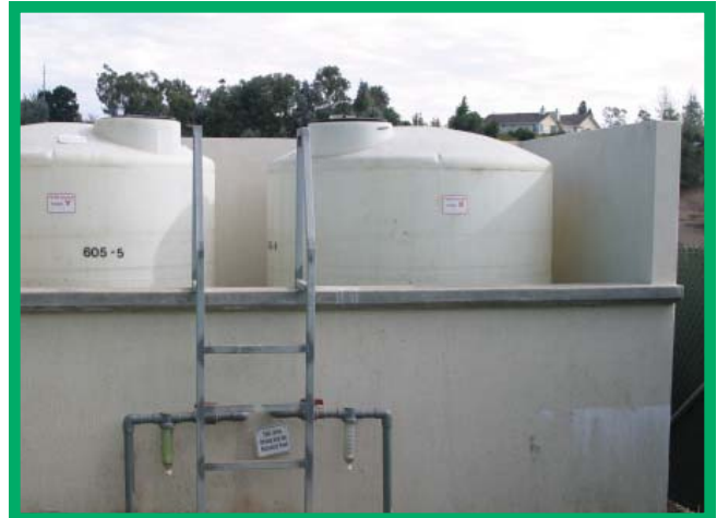
Example of secondary containment around fertilizer tanks.
