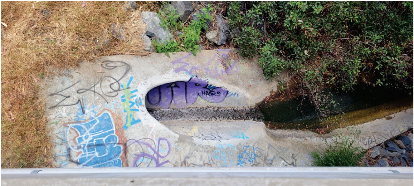
Photo 4: View of the concrete pipe culvert where the unnamed tributary to Santiago Creek originates. Photo Date May 3, 2023.
