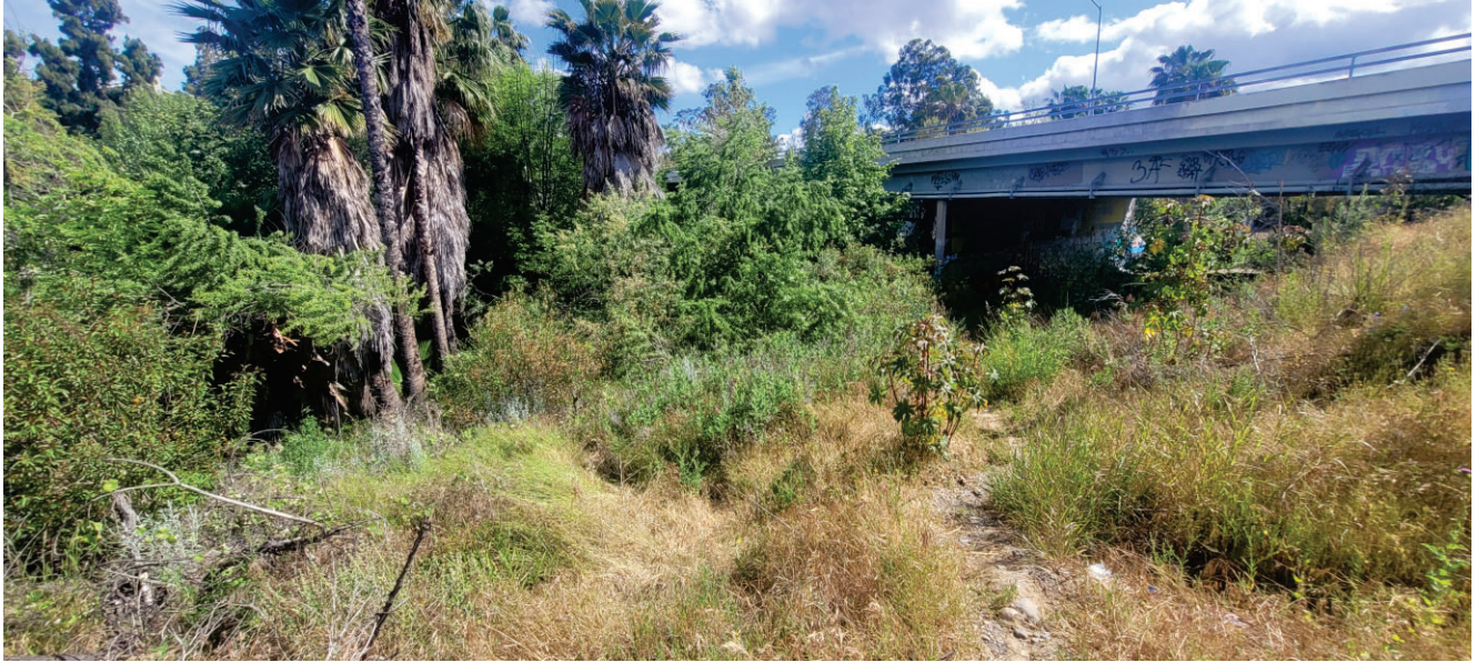
Photo 5: Looking northeast at Santiago Creek and the Cannon Street Bridge near the southern-central portion of the project site. May 3, 2023.
