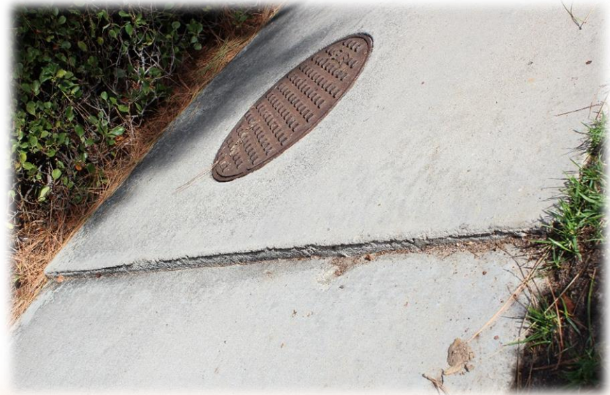
Concrete in need of work
